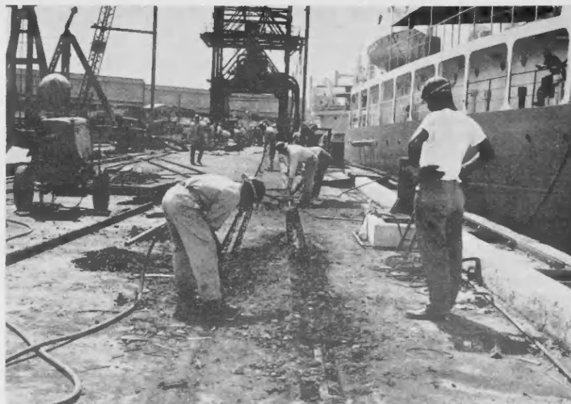
WHEN NO. 1 Finger Pier was put into service in 1949 its deck was lined with railroad tracks to accommodate the narrow-gauge train that at one time operated over a route that covered a major portion of the refinery. The train hauled supplies and equipment.
